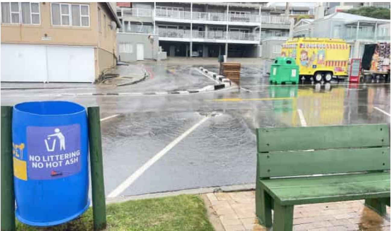
Photo 1: Surcharging Sewer Main Upstream of PS 1
