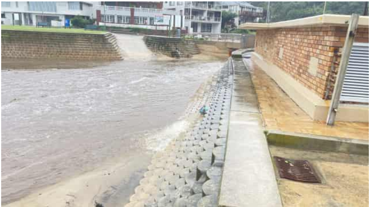
Photo 3: Emergency overflow discharging
