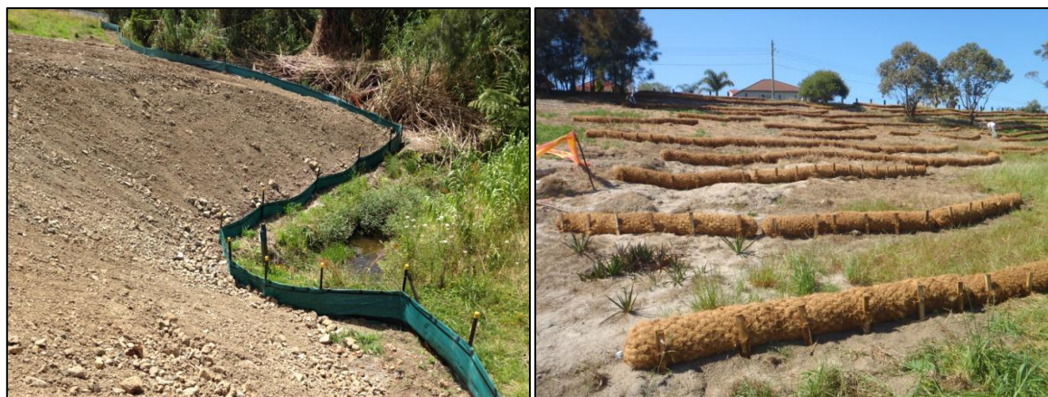
Figure 16: Examples of silt fences (left) and coir logs (right) used to trap sediment mobilised from steep slopes.
