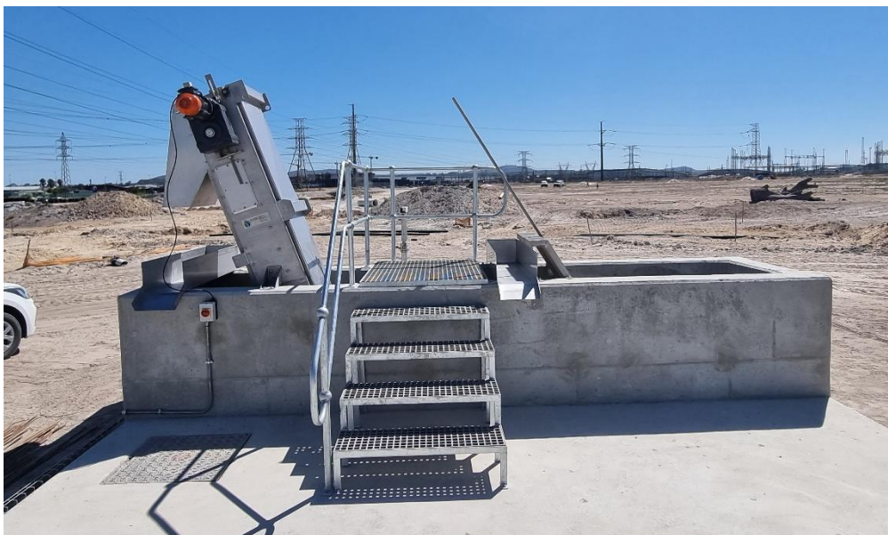
Figure 3: Concrete underground MBR Treatment Plant Inlet Works
