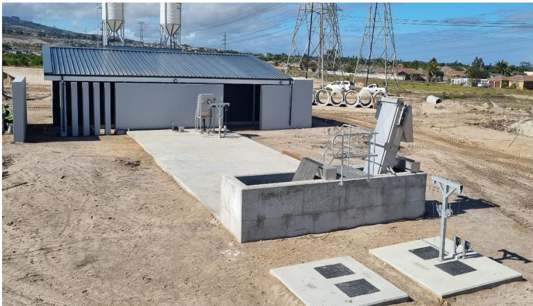
Figure 5: Recently completed MBR plant showing inlet works and control room
