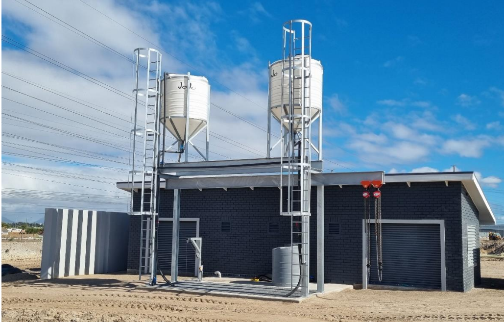
Figure 4: Concrete underground MBR equipment room and sludge silos
