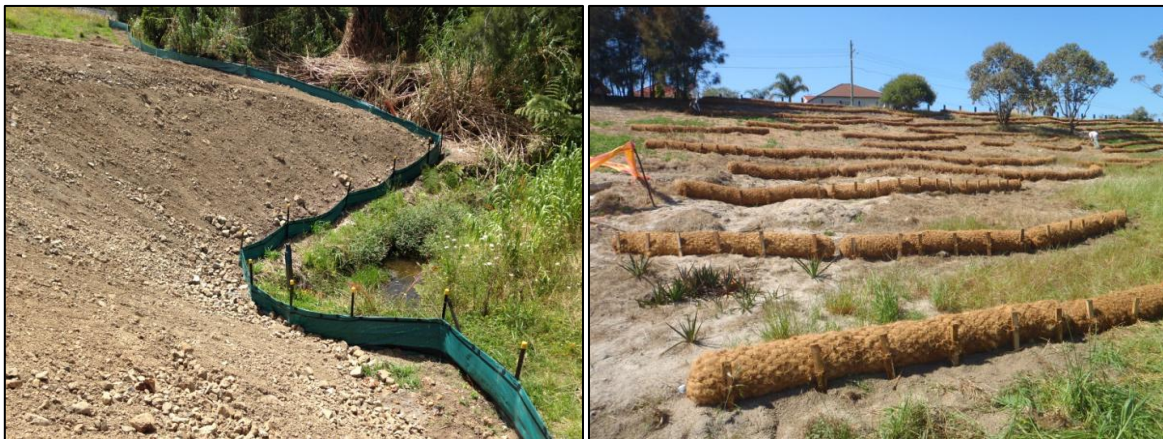
Figure 10: Examples of silt fences (left) and coir logs (right) used to trap sediment mobilised from steep slopes.
